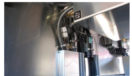
HVAC exterior compartments
